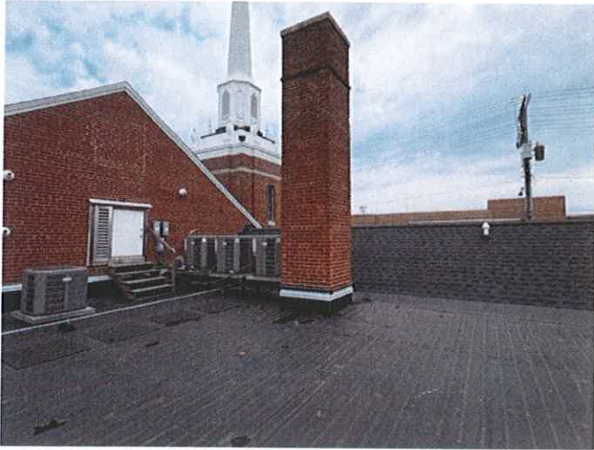
Existing brick chimney structure in need of repair.
